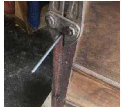
Pushed through the case to get the correct length then cut and file smooth.
