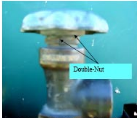
Figure 1. Leaking shutoff with a double-nut configuration
